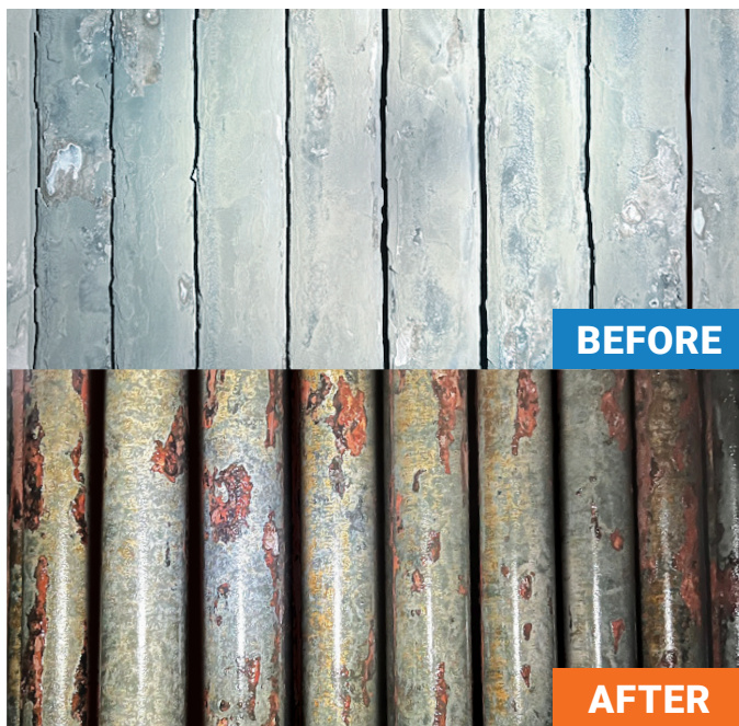
200 HP boiler showing thick scale build-up
